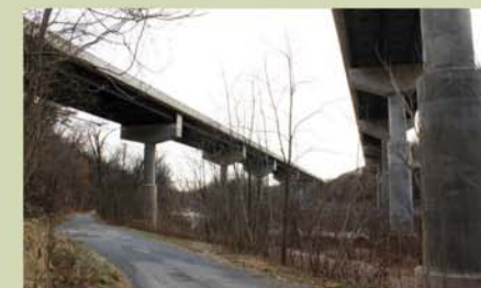
Looking southwest beneath the north and south bound I-81 bridges over SR 72 (background), Swatara Creek and Old State Road (foreground).
